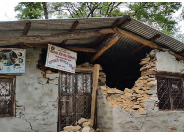
Building of a health facility damaged due to earthquake
